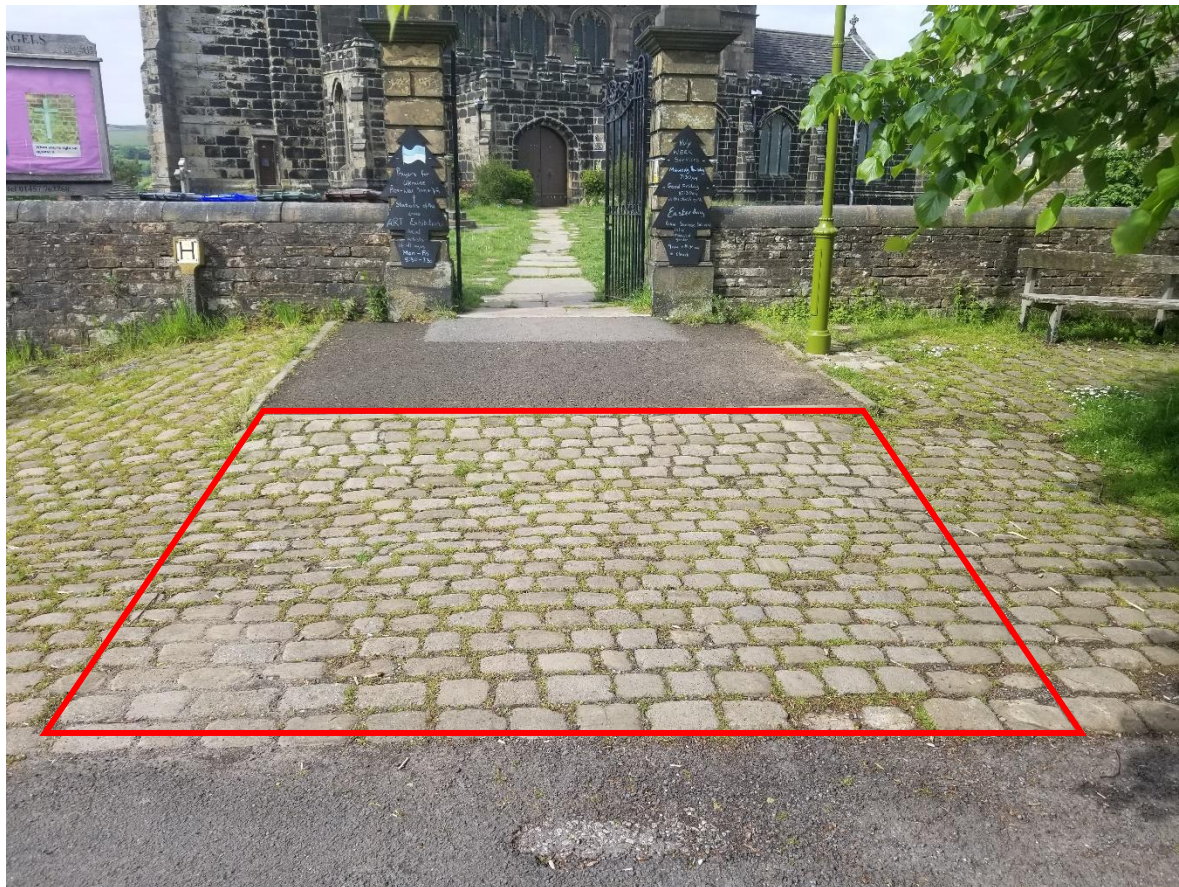
The area outside the churchyard, showing the cobbled area that is to be replaced by tarmac.
